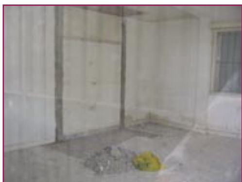
The centre needed extensive refurbishment
